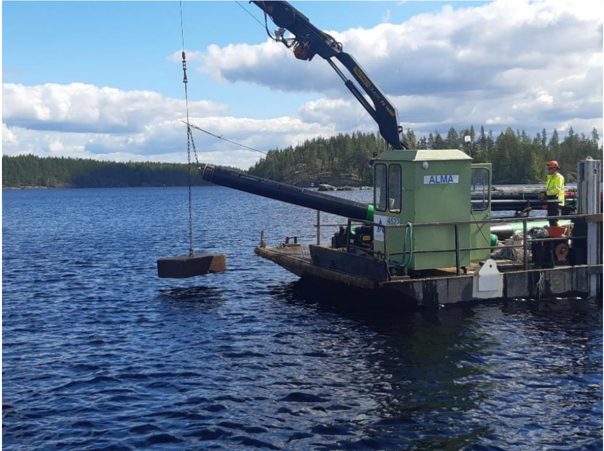
Figure 6 A weight being lowered in the water, pulling the buoy with it
